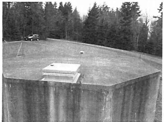
Looking at hexagonal tank
