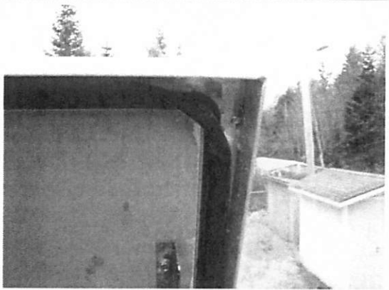
Access hatch on circular tank
