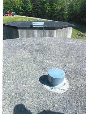
Storage tank 1 Vent
