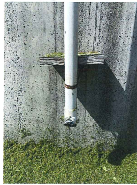
Storage Tank 2 Overflow
