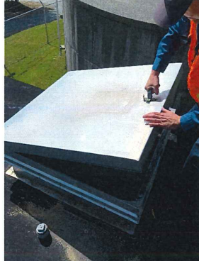
Storage Tank 2 Hatch
