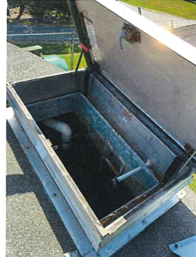
Storage Tank 1 Hatch Seal
