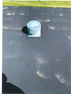
Storage Tank 2 Vent
