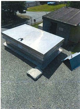
Storage Tank 1 Hatch
