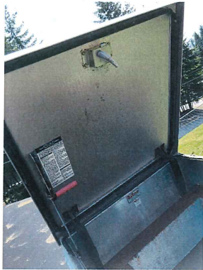
Storage Tank 2 Hatch Seal
