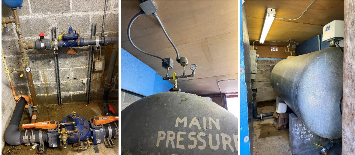
(L)PRV and other valving for distribution (Center) & (R) Hydro-pneumatic tank
