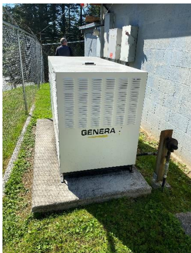
(Above) On-site generator
