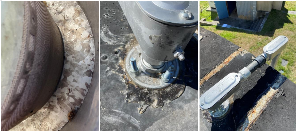
(L) Screened vent for reservoir #1 (Center) & (R) Electrical conduit for reservoir #1
