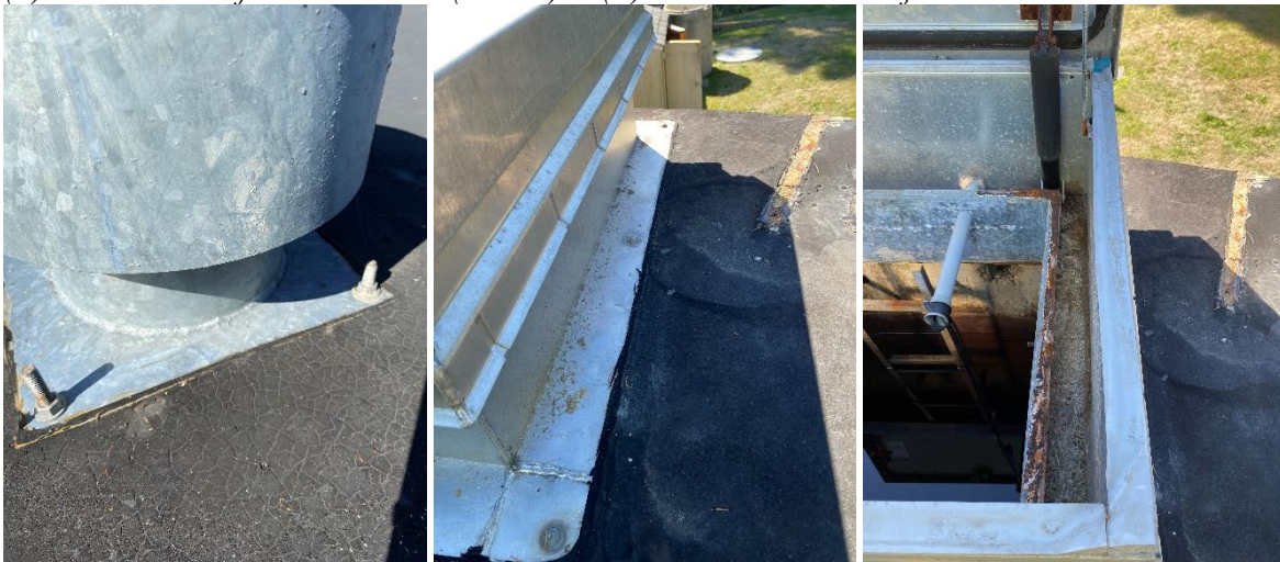
(L) Vent for reservoir #1 (Center) Hatch for reservoir #1 (R) Bottom of hatch seal for reservoir #1
