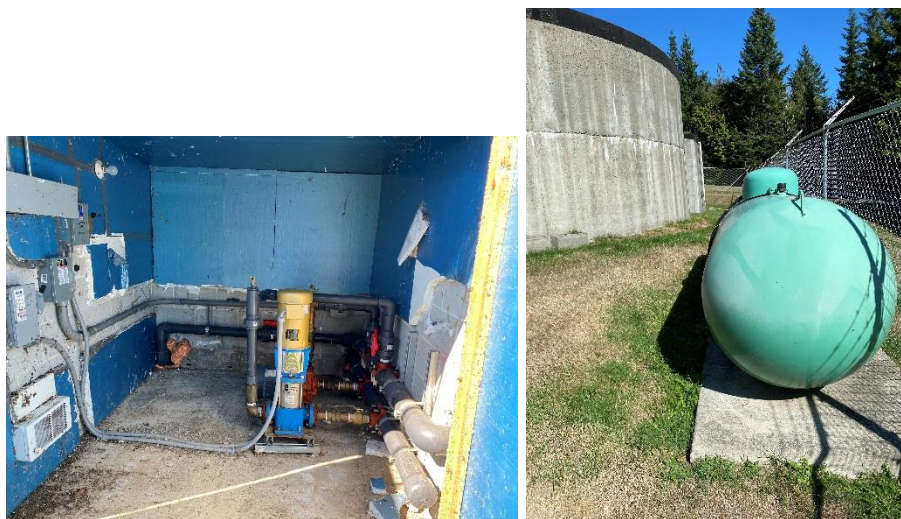
(L)Booster pumps (R) Propane tank for generator
