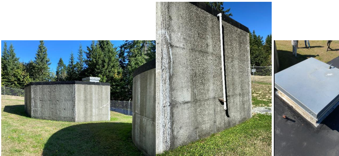
(L) Reservoir #2 (Center) Screened overflow for reservoir #2 (R) Closed hatch for reservoir #2
