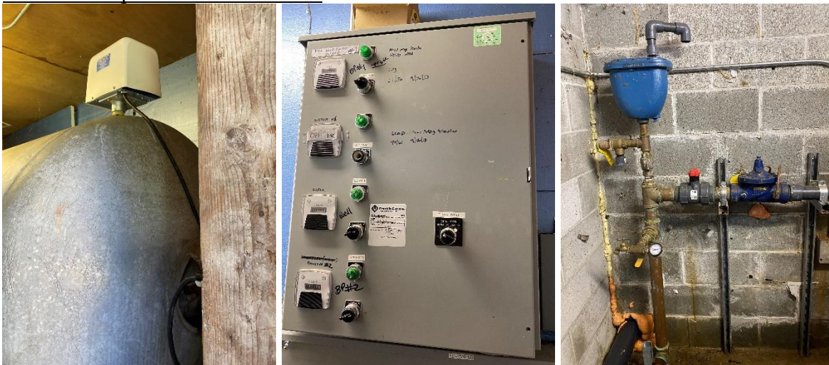
(L) Air compressor on hydropneumatic tank (Center) Electrical controls (R) PRV
