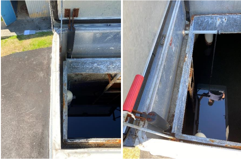
(L) Hatch seal for reservoir #1 (R) Hatch seal for reservoir #1
