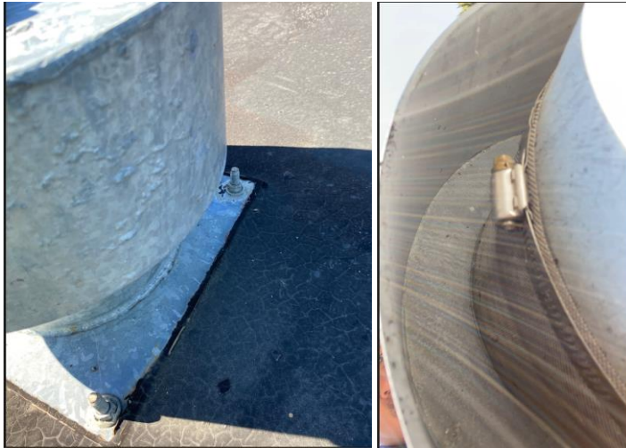
(L) Vent for reservoir #2 (R) Screened vent for reservoir #2
