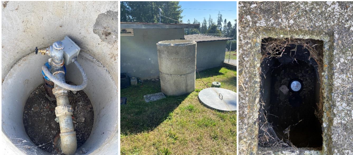
(L) Well #1 & sample tap (Center) Well #1 with concrete structure protecting wellhead (R) Source meter
