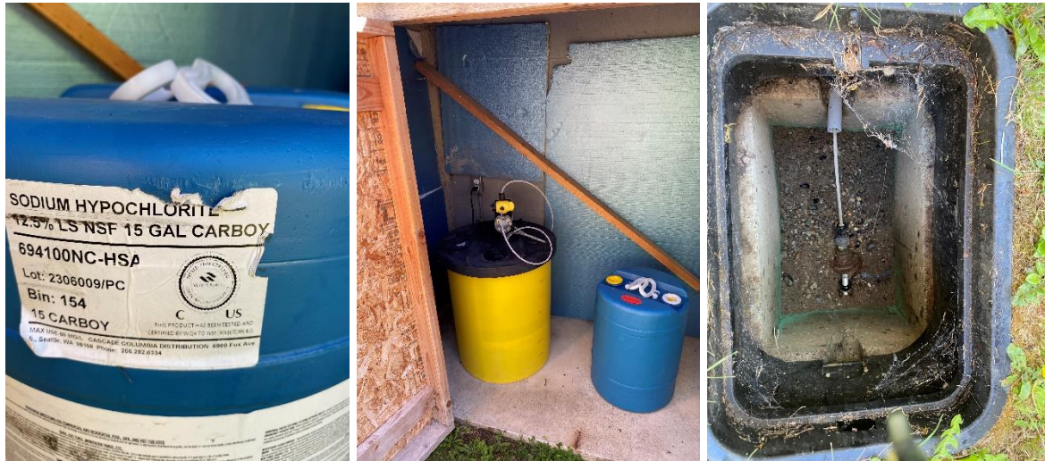
(L) Sodium hypochlorite NSF (Center) Chlorine solution tank and feed pump (R) Chlorine injection point
