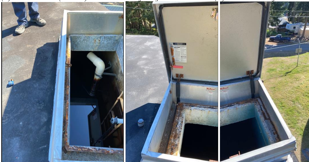
(L) Open hatch and water inlet for reservoir #2 (Center) & (R) Hatch seal for reservoir #2
