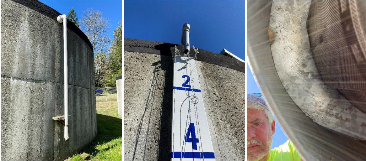
(L) Screened overflow on reservoir #1 (Center) Open end on tank level for reservoir #1 (R) Screened vent for reservoir #1
